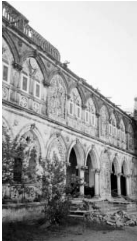
Fig. 10.1 Increase in seismic damage with height in a stone masonry building, Gujarat, India, 2001
